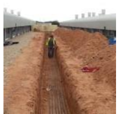
Cable trench at Baulker Farm
